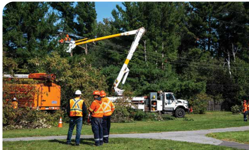
Image 18: Fallen power lines and light stands (left); Tree trimming (right)
