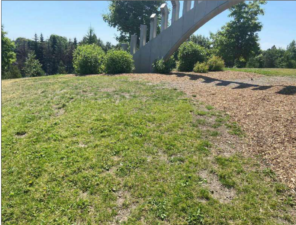
Photo 3: East Berm: Areas of bare soil were observed at the top of the berm.
