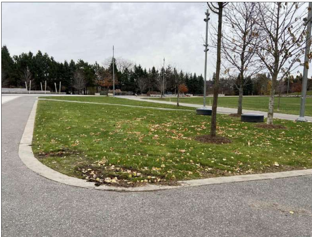
Photo 16: Former Eastern Landfill: Tire ruts were observed near the west end of the grassed area south of the Water Jet Plaza.
