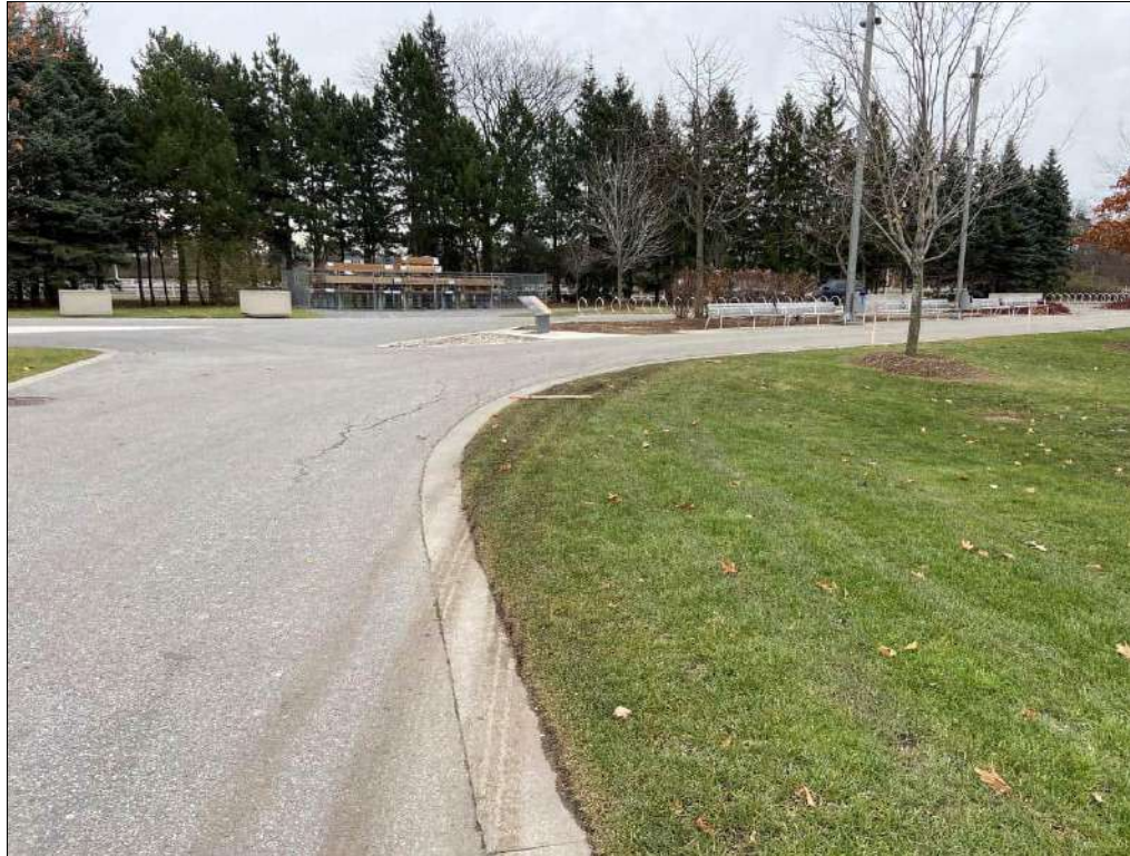
Photo 17: Former Eastern Landfill: Tire ruts were observed at the northeast end of the Great Lawn.
