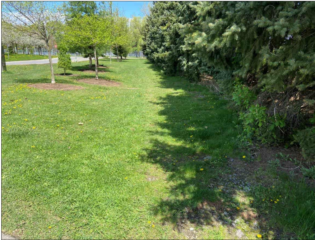
Photo 23: Eastern Perimeter Drainage Swale: General view of the swale east of the Ice Rink and Heirloom Orchard. Small areas of bare soil were observed in the area of the utility trench previously excavated within the swale.
