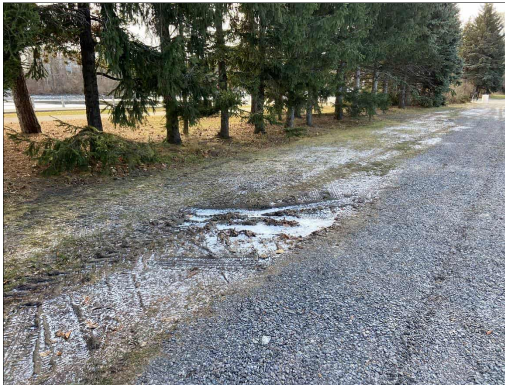
Photo 21: Former McElroy Building/Eastern Perimeter Drainage Swale: Areas of bare soil, stressed vegetation and tire ruts on either side of the gravel covered portion of this area.
