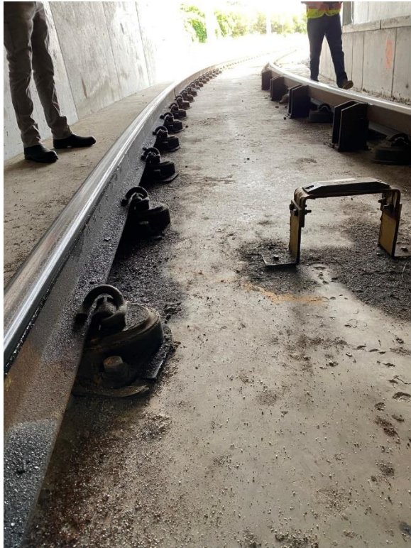
Figure 4.17: Grease Contamination at East Connector
