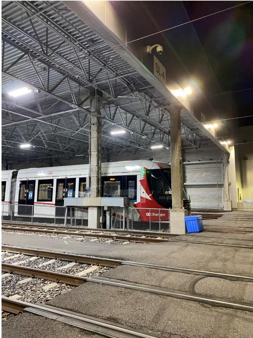
Figure 4.12: Lack of Doors at Storage Shed
