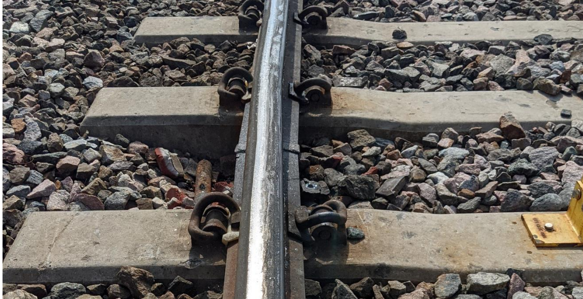
Figure 4.21: Kinks at Weld Location (C19), Including Grease Contamination of the Top of Rail
