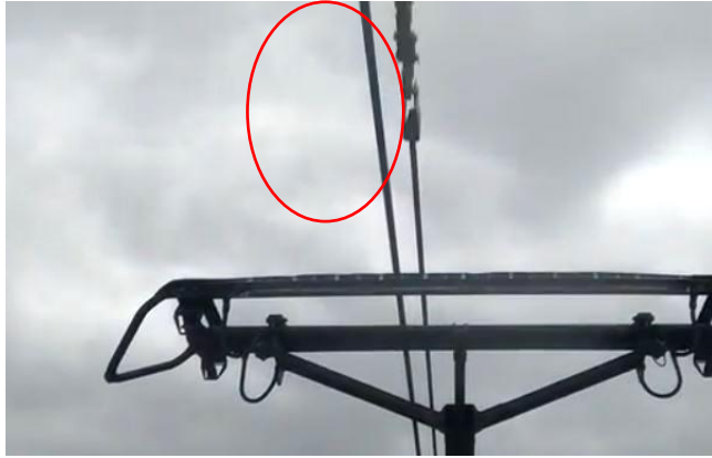
Figure 3.39: Messenger Wire Cut-in Insulation
