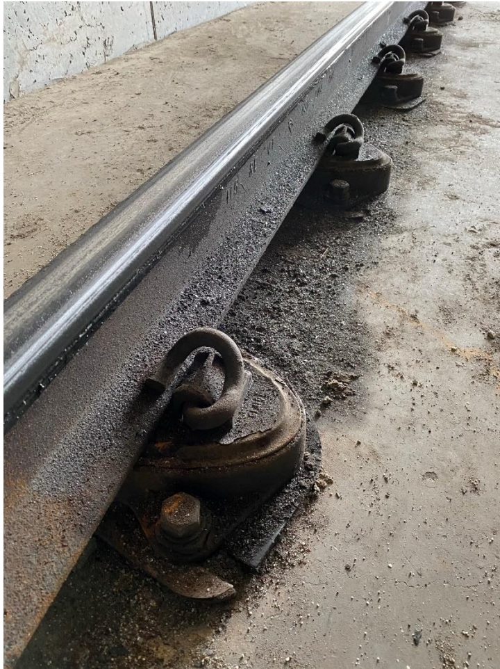
Figure 5.6: Manual Grease Application Location at East Connector Tunnel
