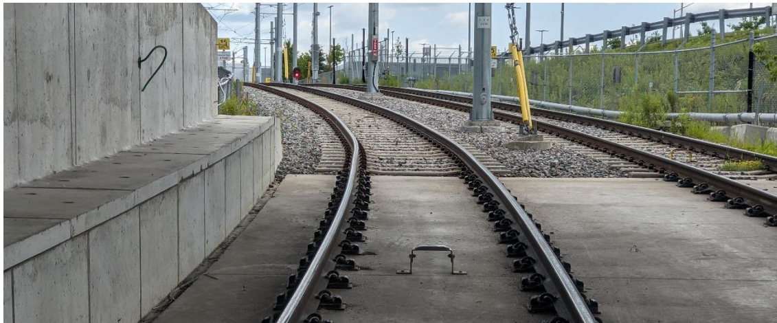
Figure 4.22: EB Connector, Track Geometry at Interface Between Ballast Track and DFF Track
