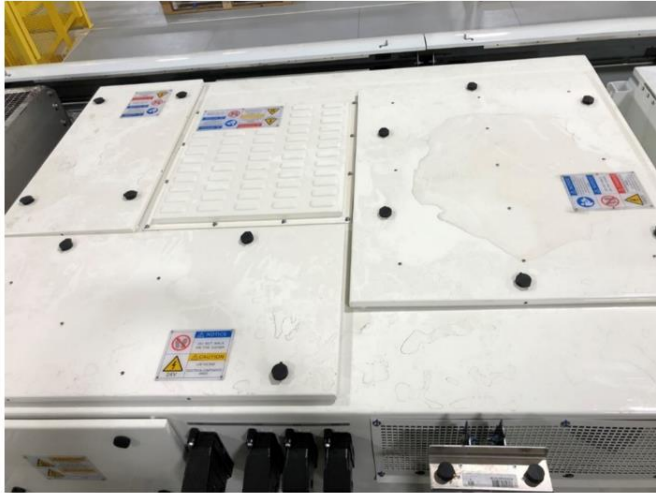
Figure 3.83: Previously Used Traction Converter Installed on LRV1152
