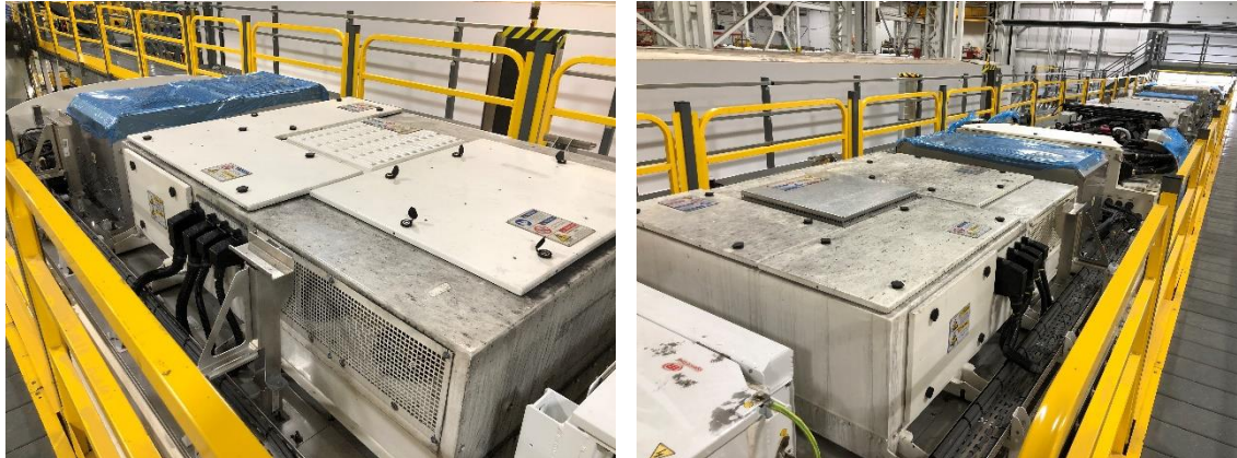
Figure 3.58: Examples of traction converter containers at Brampton
