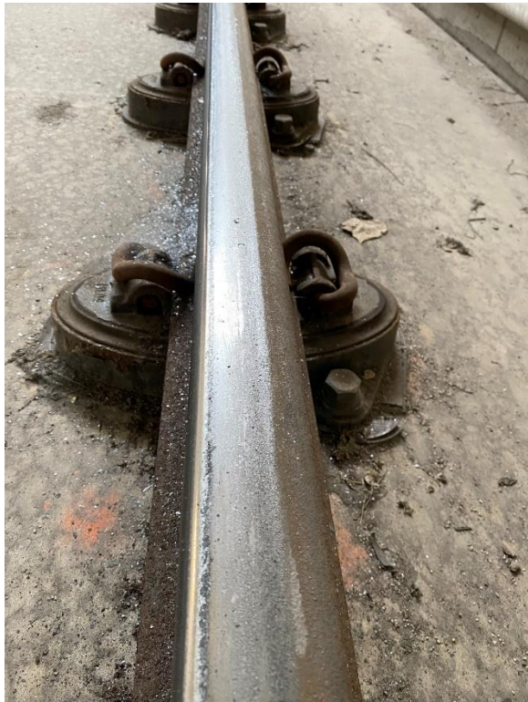
Figure 5.8: Less Grease on Rail Elsewhere in the Connector Tunnel
