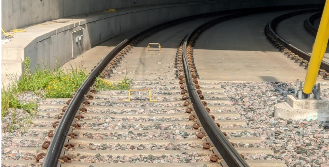
Figure 4.23: WB Connector, Track Geometry at Interface Between Ballast Track and DFF Track
