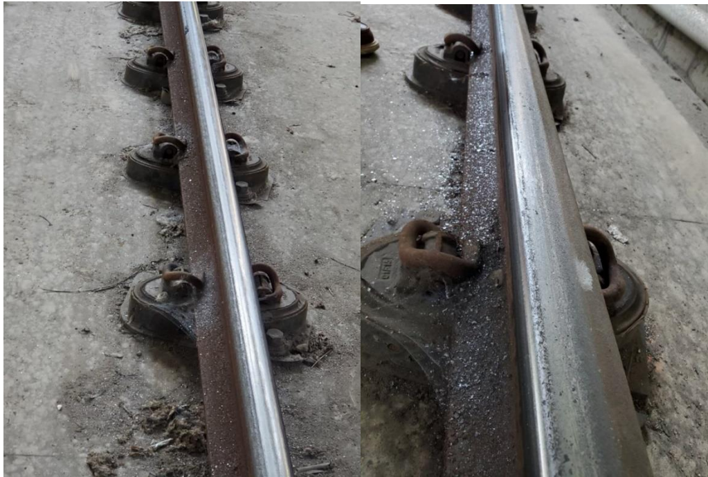
Figure 5.10: Metal Shaving at East Connector Portal Tunnel
