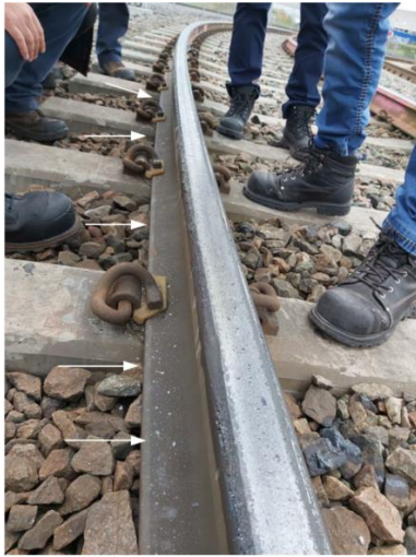
Figure 5.1: Metal Shavings Along Rail Curve 19
