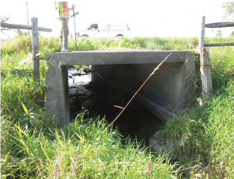
Photograph 8 Looking upstream (south) at downstream face of the Corkstown Road 3.0 meter span by 2.0 meter rise open bottom box culvert
