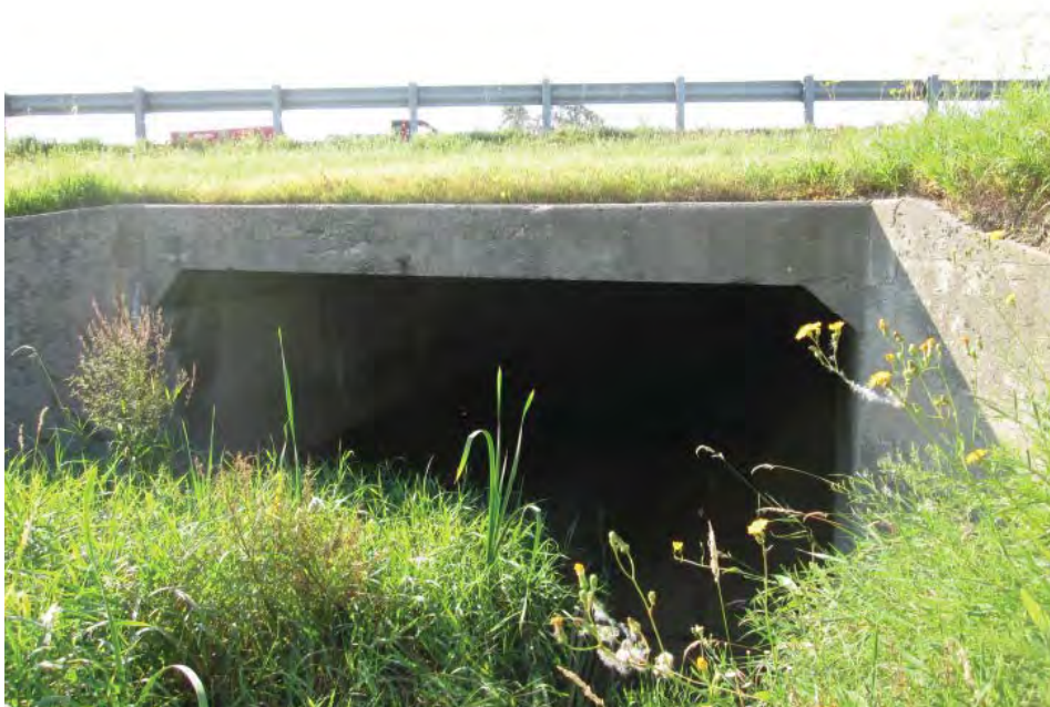
Photograph 2 Looking north at downstream face of the Highway OR 417 4.9 meter span by 2.1 meter rise open bottom box culvert
