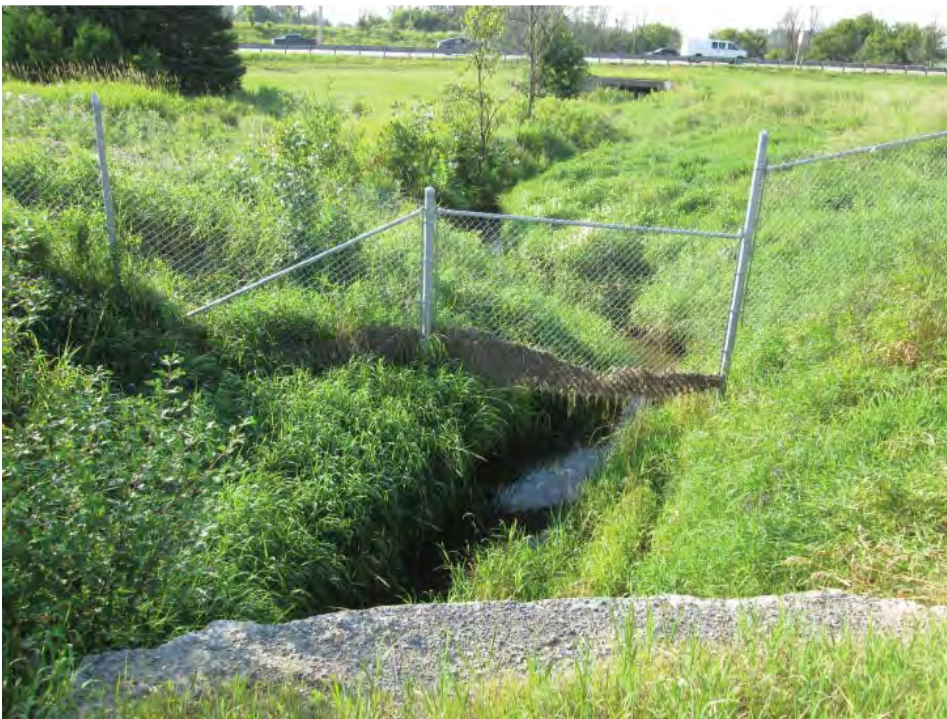
Photograph 6 Looking upstream (south) from the Corkstown Road 3.0 meter span by 2.0 meter rise open bottom box culvert towards Highway OR 417
