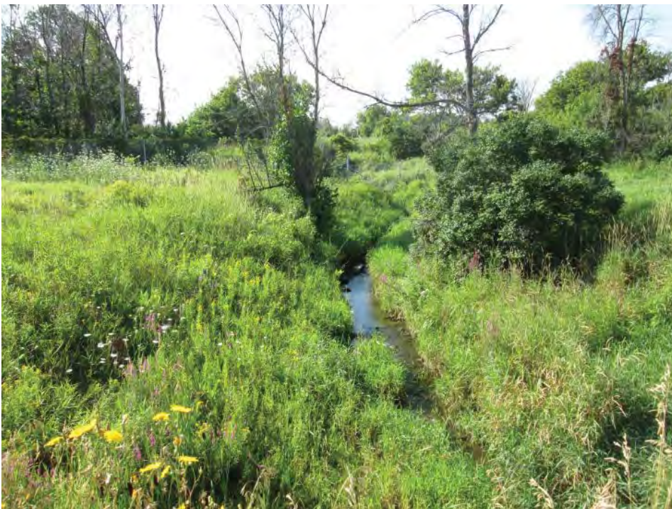
Photograph 10 Looking downstream (north) from the Corkstown Road 3.0 meter span by 2.0 meter rise open bottom box culvert
