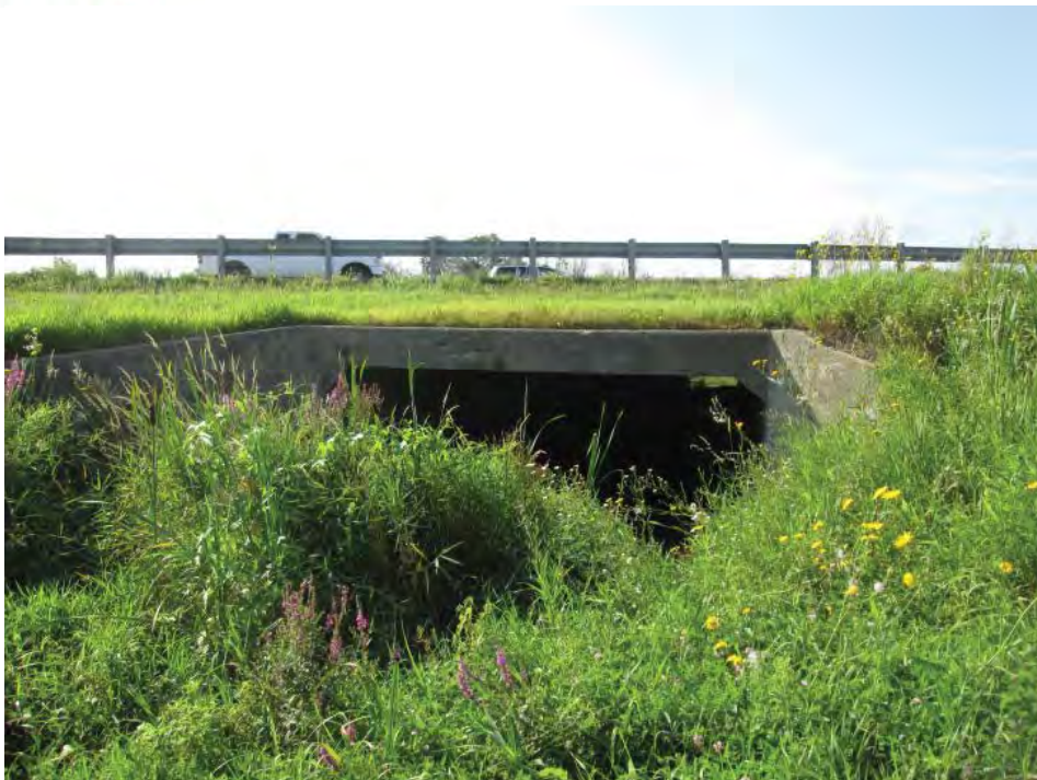
Photograph 1 Looking north at downstream face of the Highway OR 417 4.9 meter span by 2.1 meter rise open bottom box culvert
