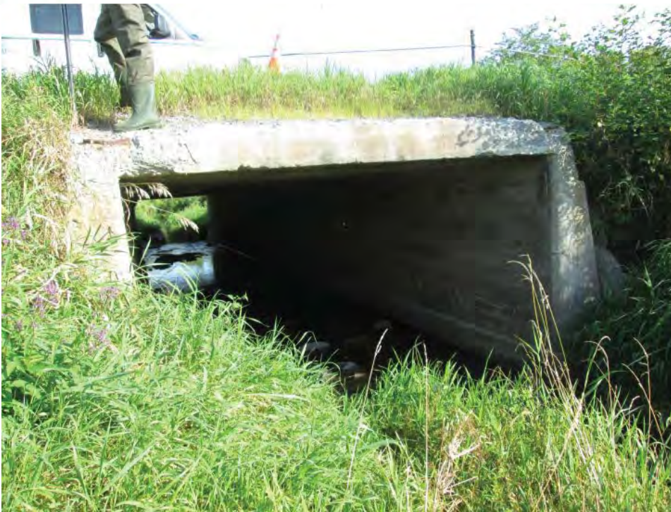
Photograph 7 Looking downstream (north) at upstream face of the Corkstown Road 3.0 meter span by 2.0 meter rise open bottom box culvert
