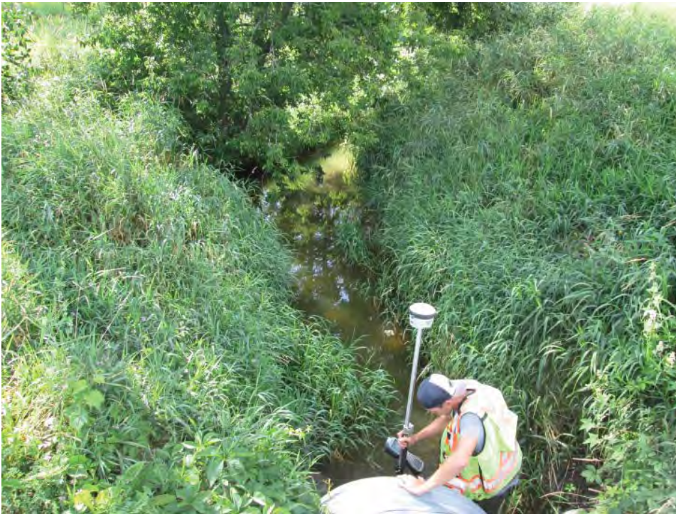
Photograph 13 Looking upstream (south) from the 1200 mm corrugated metal pipe under the Wesley Clover Farms path
