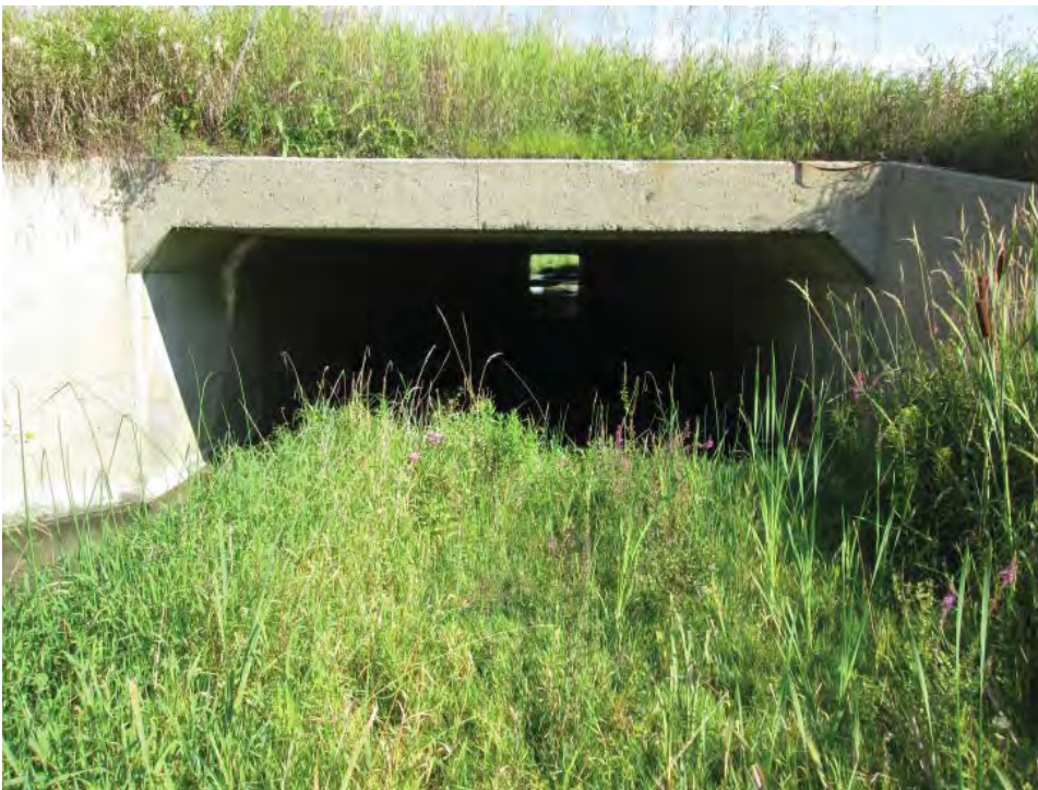
Photograph 4 Looking south at upstream face of the Highway OR 417 4.9 meter span by 2.1 meter rise open bottom box culvert
