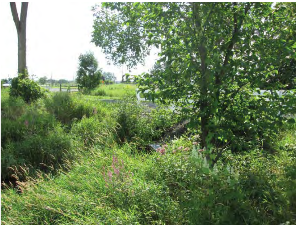
Photograph 15 Looking upstream (south) at the downstream face of the 1200 mm corrugated metal pipe under the Wesley Clover Farms path
