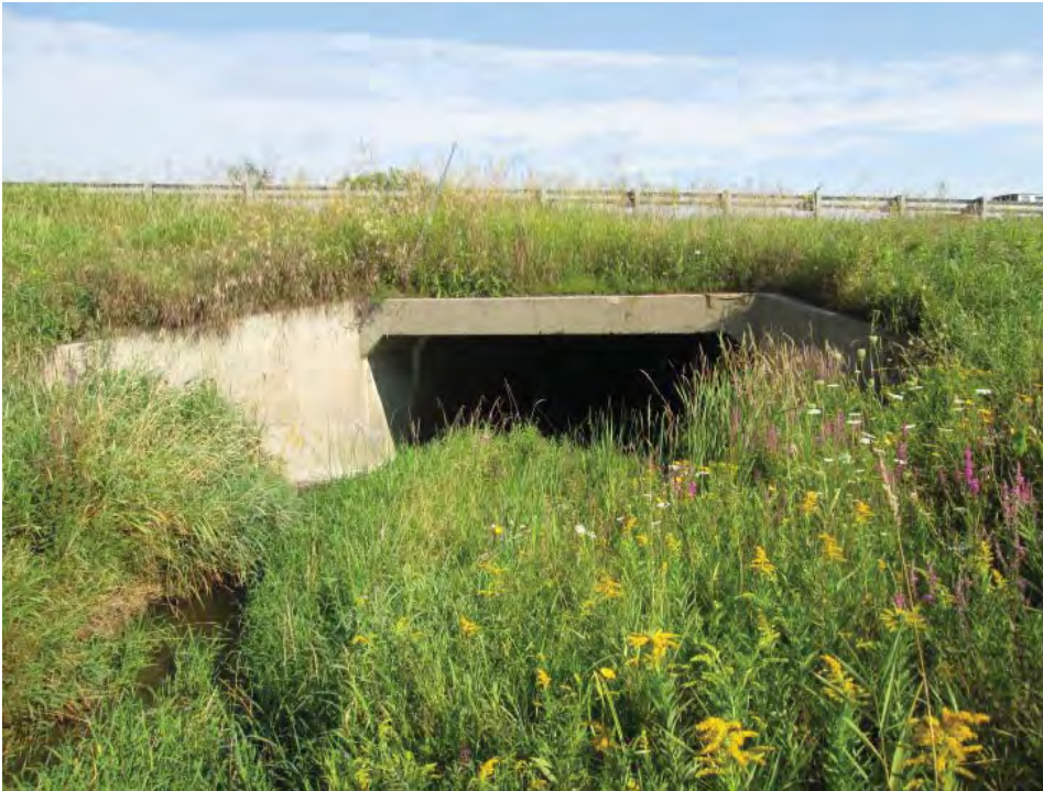
Photograph 5 Looking south at upstream face of the Highway OR 417 4.9 meter span by 2.1 meter rise open bottom box culvert
