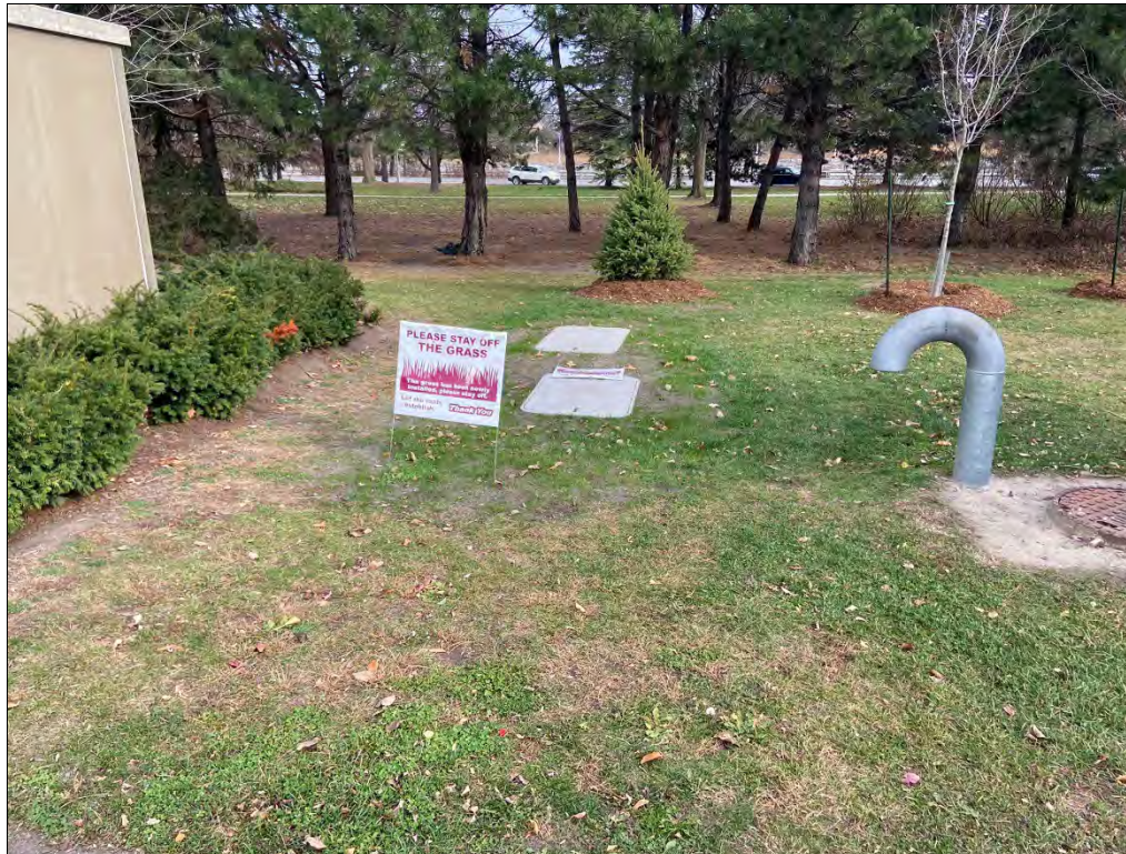
Photo 15: Former Eastern Landfill: Recent excavation to install in ground utility boxes disturbed the cover east of the Children's Garden.
