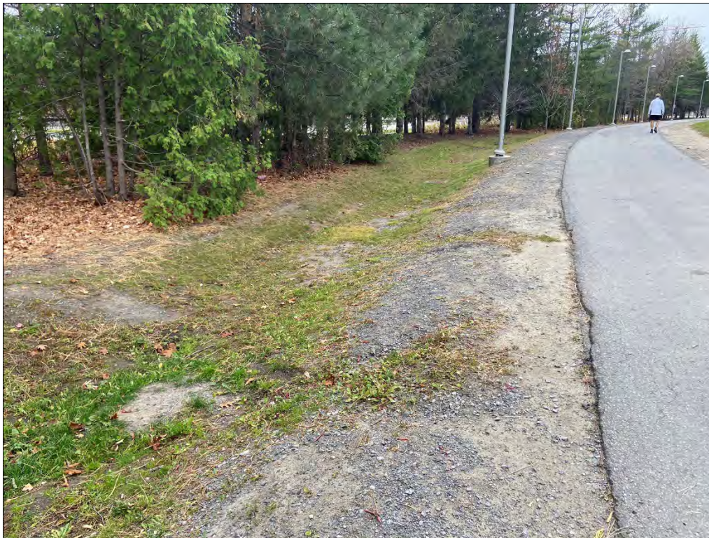
Photo 10: South Drainage Swale: General view of the swale. Road base material has eroded into the swale.
