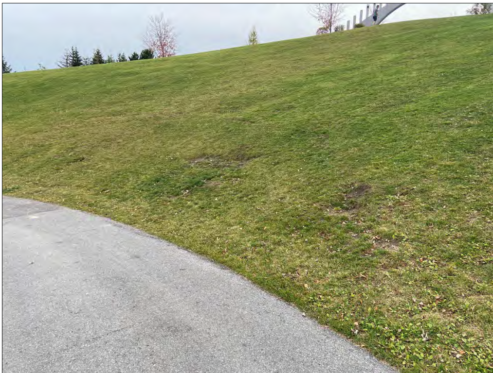
Photo 2: East Berm: General view of the steeper sloped areas along the pedestrian pathway on the east side of the berm. Note small areas of bare soil.
