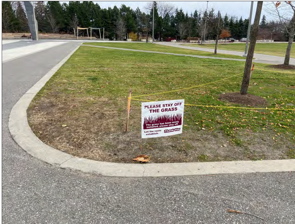
Photo 17: Former Eastern Landfill: Area of bare soil and stressed vegetation under repair southwest of Water Plaza.
