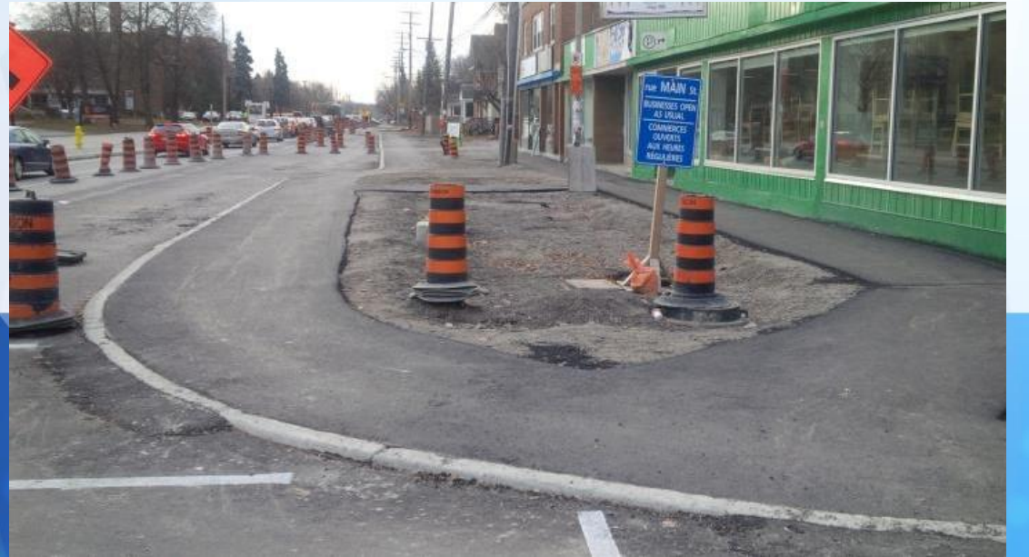
Example of providing safe and accessible travel path for pedestrians through the construction site
