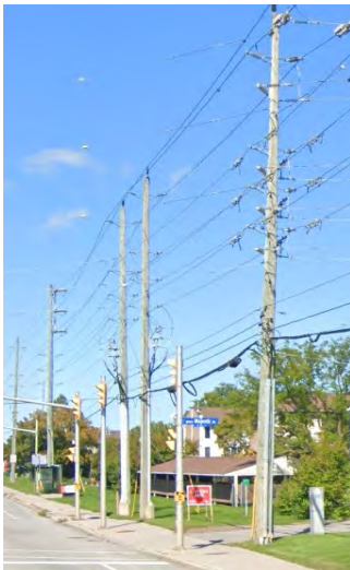
Figure 6-3 Hydro Lines on the East side of Woodroffe Avenue at Majestic Drive
