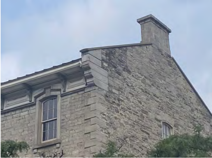
Figure 44: Historic stone chimney at the rear of 541 Sussex Drive, as seen from George Street.
