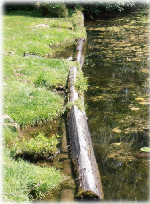
Before: Failed retaining wall and active erosion
