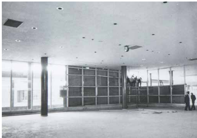
The aftermath of a sonic blast on the Air Terminal at Uplands Airport, 1960s Ingenium/Canada Aviation and Space Museum, William A. Ramsay Fonds
