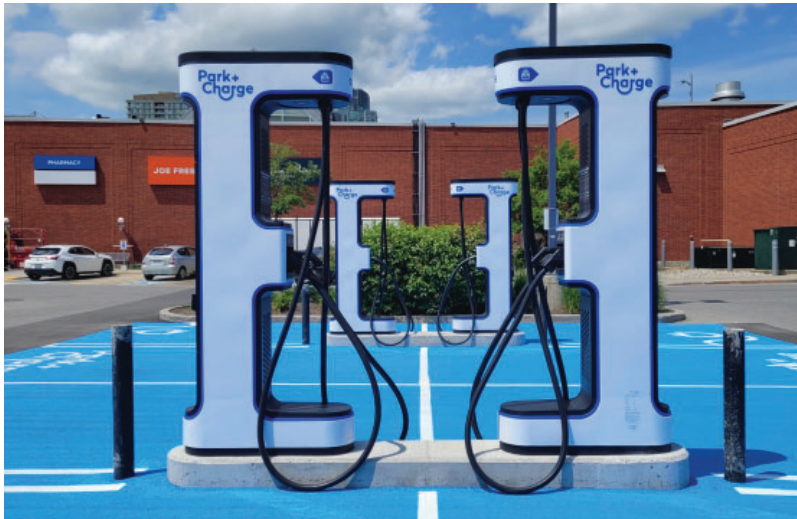
Figures 19: Provision of electric vehicle charging station along the parking.
