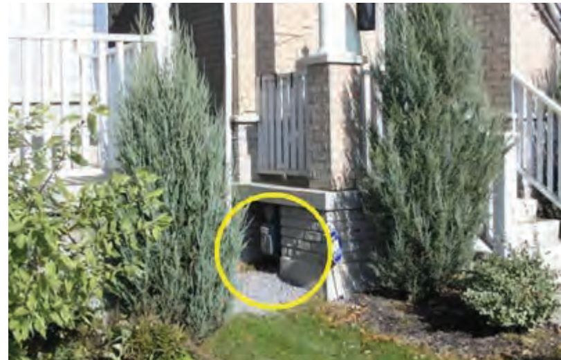
Figure 46: This utility meter is hidden from the streetscape by incorporating it into the design of the stairs.
