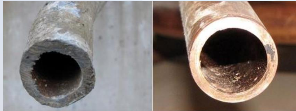
Lead Pipe (Left) & Copper Pipe (Right)
