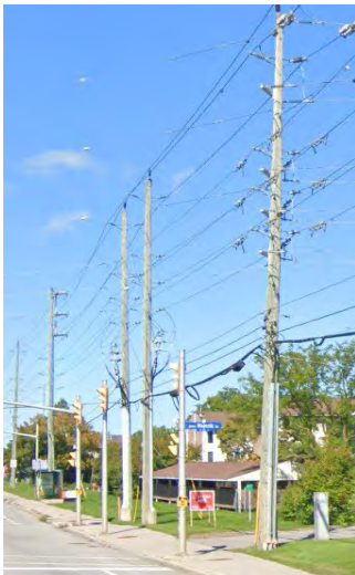
Figure 6-3 Hydro Lines on the East side of Woodroffe Avenue at Majestic Drive
