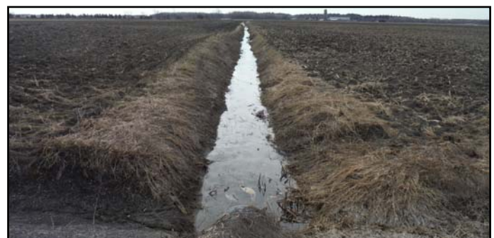
Channelized drainage feature on Regimbald Road
