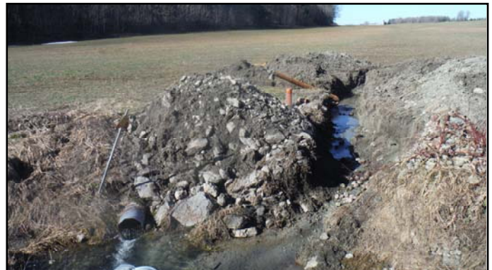
Headwater drainage feature that could benefit from tile outlet control in the Becketts Creek catchment
