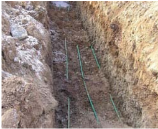
Figure 26: Installation of a geothermal ground loop system shows the pipes that, with the aid of an indoor pump, will move heat into or out of the earth to heat or cool a home (installation for a home near Munster).
